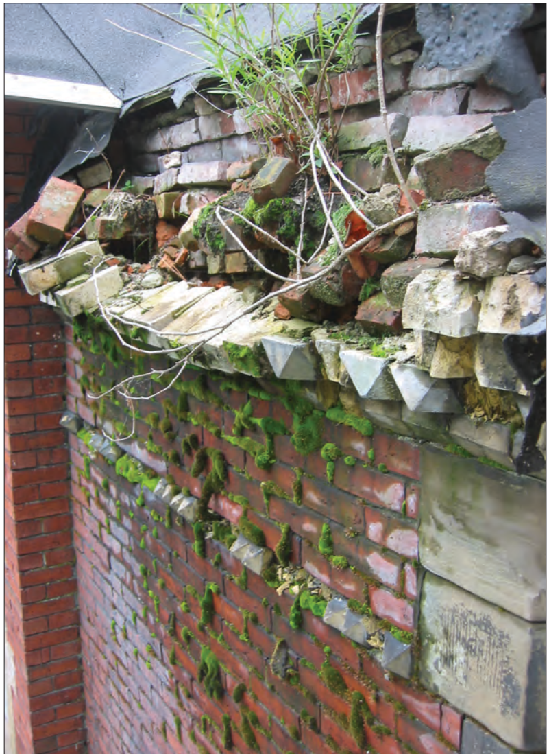
Fig. 1. Mortar failure at Pine Bank Mansion, Boston, Massachusetts, 2004. This mass brick masonry was set with lime mortar that has failed due to decades of water infiltration and freezing and thawing. It is an example of the type of sacrificial-joint softening failure that occurs with older, lower-strength mortar binder materials. All figures by author.
